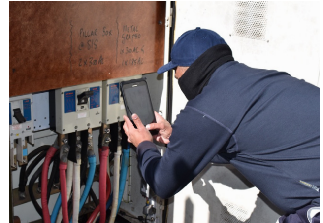
City of Cape Town official capturing performance data at a minisubstation for electricity asset management use case
